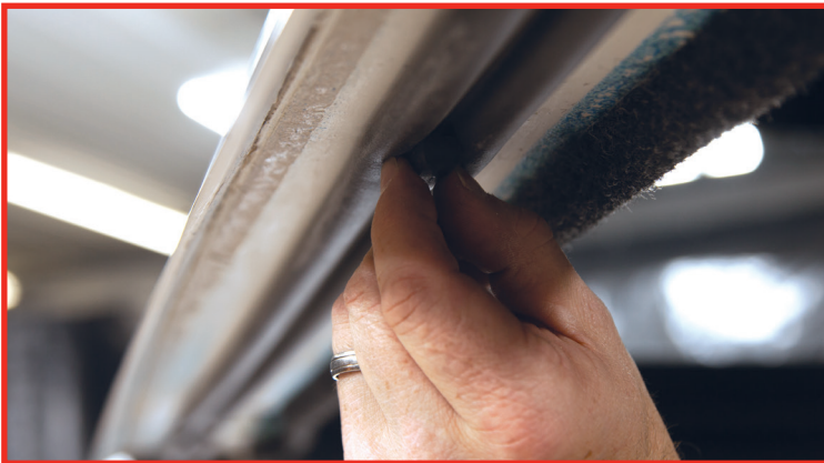
Remove (4) spacers tucked into the bulb seal, on the underside of the cap sill.
