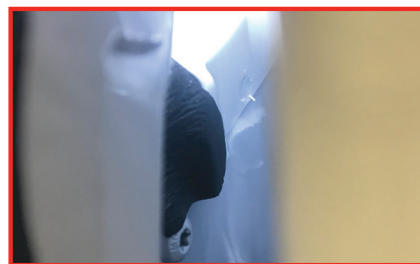
Locate gap in front of bed. Cut and place a 2" piece of putty/butyl tape over gap.
